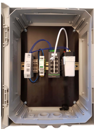
Fig. 6. INSIDE Connect in electrical cabinet with switch
